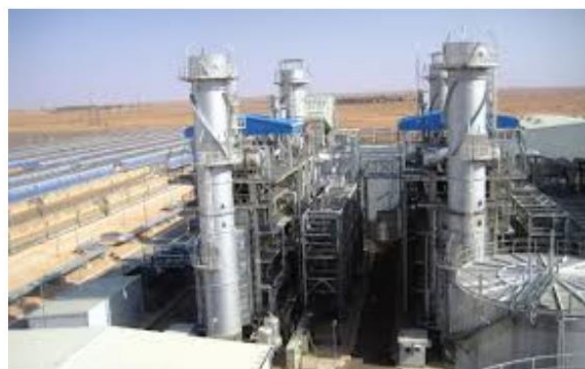
Fig. 6. Hybrid power plant near Hassi R'Mel in Laghouat
