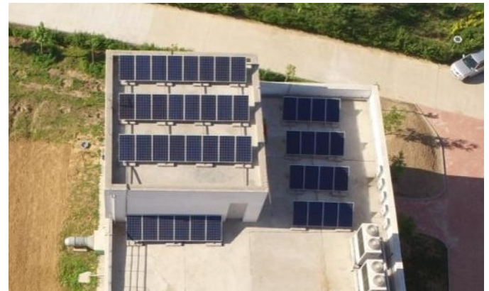
Fig. 6. Photovoltaic power generation project case site.
